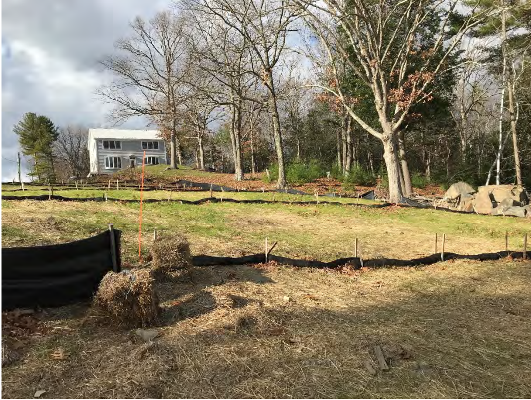
Fig 1: Slope above the cable house at the Eversource property/west side of the bay. Viewing northwest. (11-17-20)
