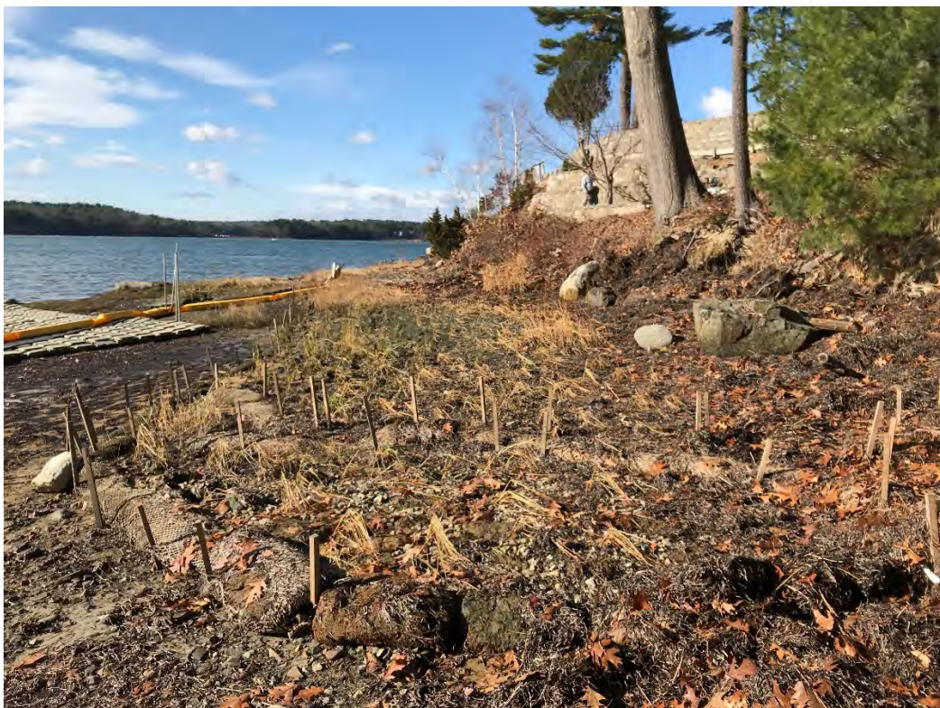
Fig 6: Salt marsh restoration at Gundalow Landing/east side of the bay. Viewing northwest. (11-17-20)
