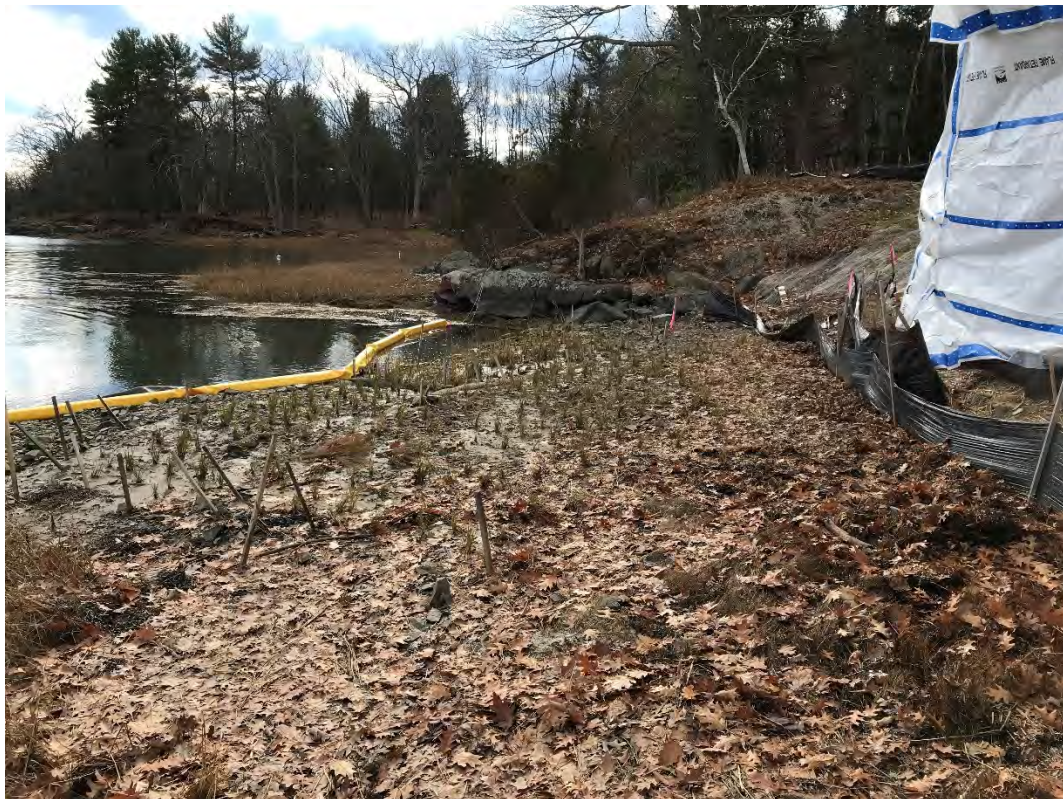
Fig 2: Toe of the slope and salt marsh restoration at the Eversource property/west side of the bay. Viewing southeast. (11-17-20)
