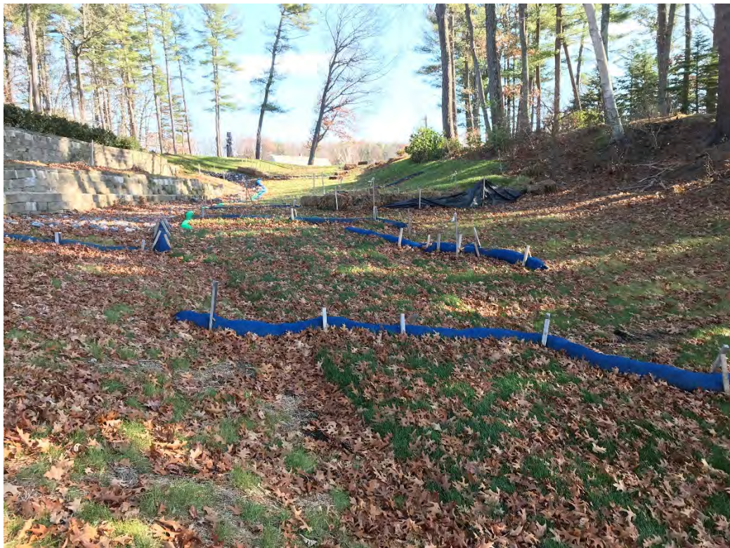
Fig 4: Slope below the manhole at Gundalow Landing/east side of the bay. Viewing east. (11-17-20)
